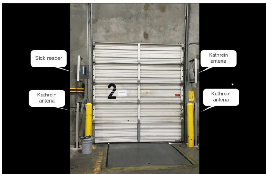
Figure 5. RFID infrastructure in receiving dock
